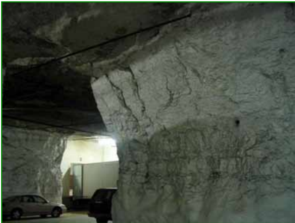
Figure 7-21 – Pillar Ground Control Problems Resulting from Curved Pillars
