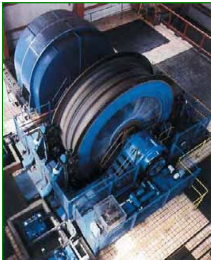
Figure 4-3 – Tower-mounted Koepe Hoist
