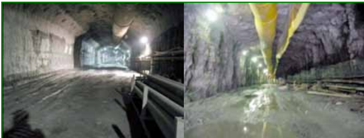
Figure 7-28 – Overbreak comparison of two separate contracts in the same rock conditions [R75]
